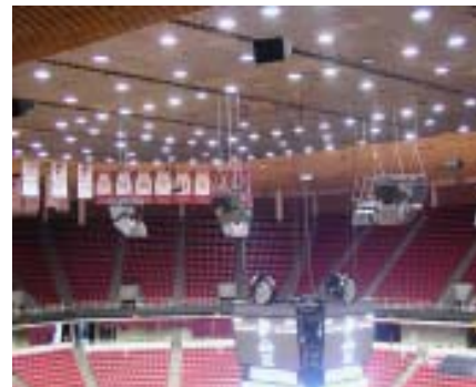
SPL Integrated Solutions designed and installed a new audio system at the Hilton Coliseum with JBL Professional PD5000 Series loudspeakers
