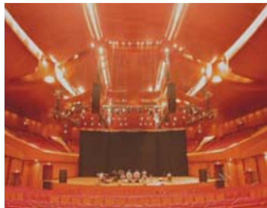
Madema's JBL VERTEC VT4888 system installed in the 2,800 seat performance hall at Rome's Parco della Musica.
