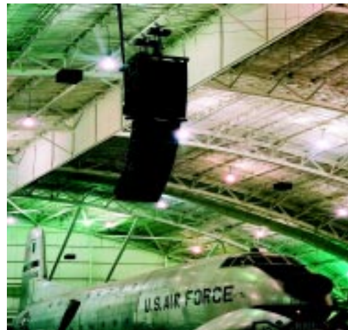
Suspended array of JBL VT4880 subwoofers and VT4888 midsize line-array elements in the United States Air Force Museum at Wright-Patterson AFB in Dayton Ohio, part of the multi-array system installed by Washington Professional Systems
